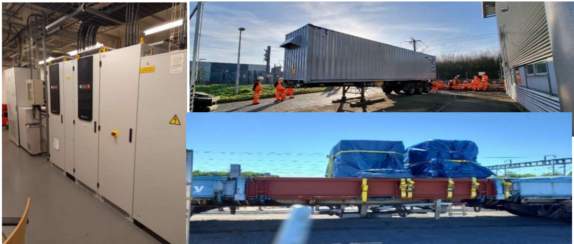
FIGURE 18 - STRATFORD UPS INSTALLATION AND TEMPORARY UPS AT SIMD
